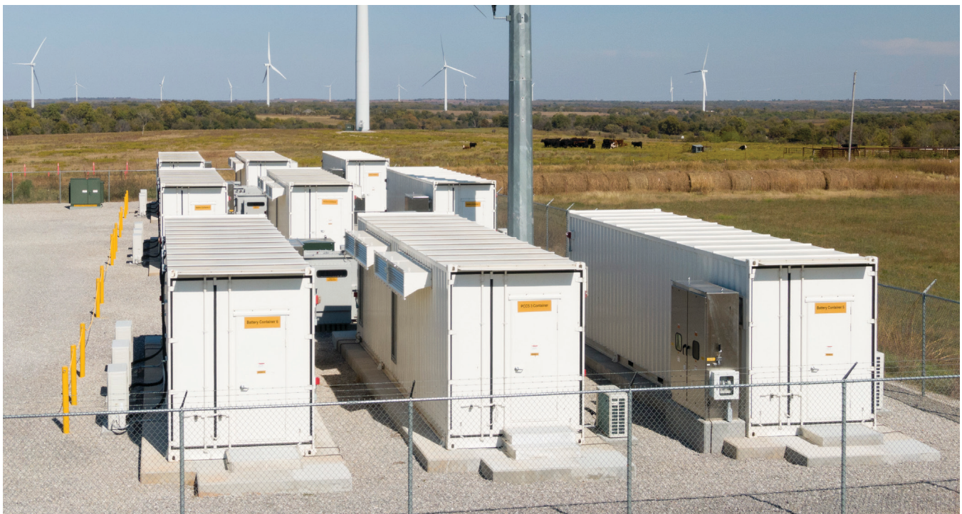
Rush Springs Energy Center is the first battery energy storage system in Oklahoma and the first energy center of its kind in the region's Southwest Power Pool (SPP). This wind and storage hybrid project generates 125 megawatts (MW) of wind energy and has a 10-MW/20 MWh battery energy storage system.
