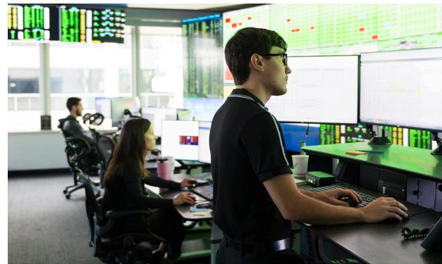
The NextEra Energy Resources Renewable Operations Control Center in Juno Beach, Florida, provides remote operations support to NextEra Energy Resources' wind, PV solar and energy storage sites.
